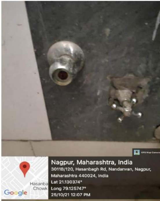
Some cocks to be replaced by push buttons
