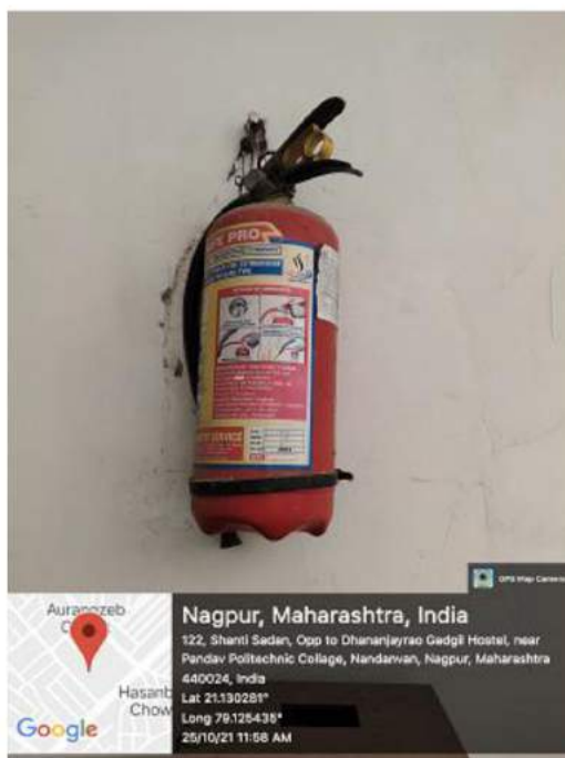
Fire Extinguisher in college
