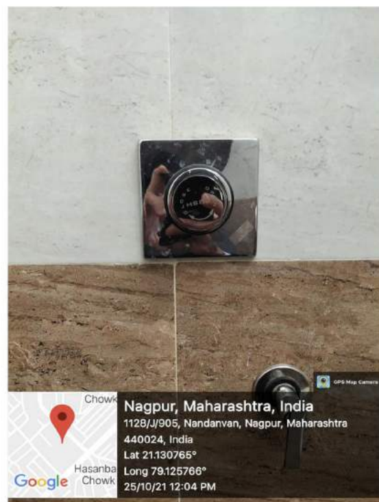
Push buttons fitted in some washrooms
