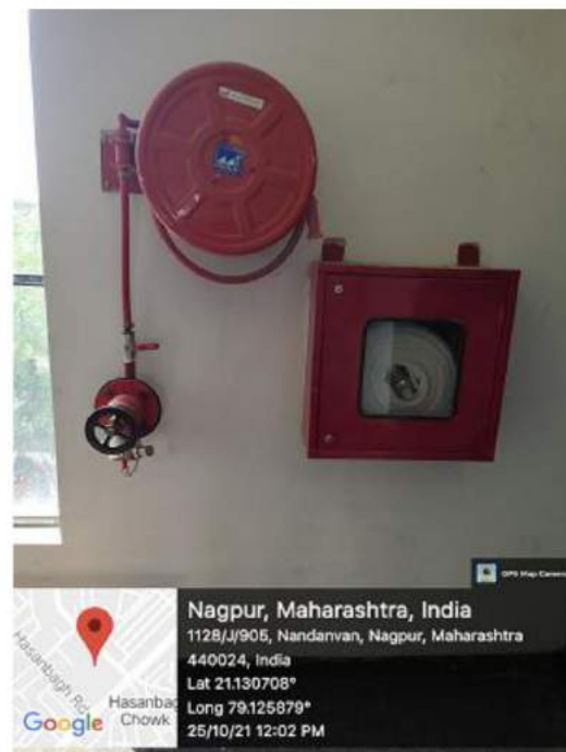
Fire Fighting system in college
