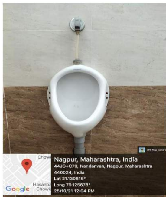
Flush to be replaced by push buttons
